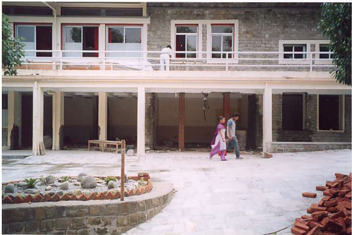
View of reconstructed front openings of Patients reception and examination rooms (Aluminium Doors & Windows will be installed there) (View from East side)
