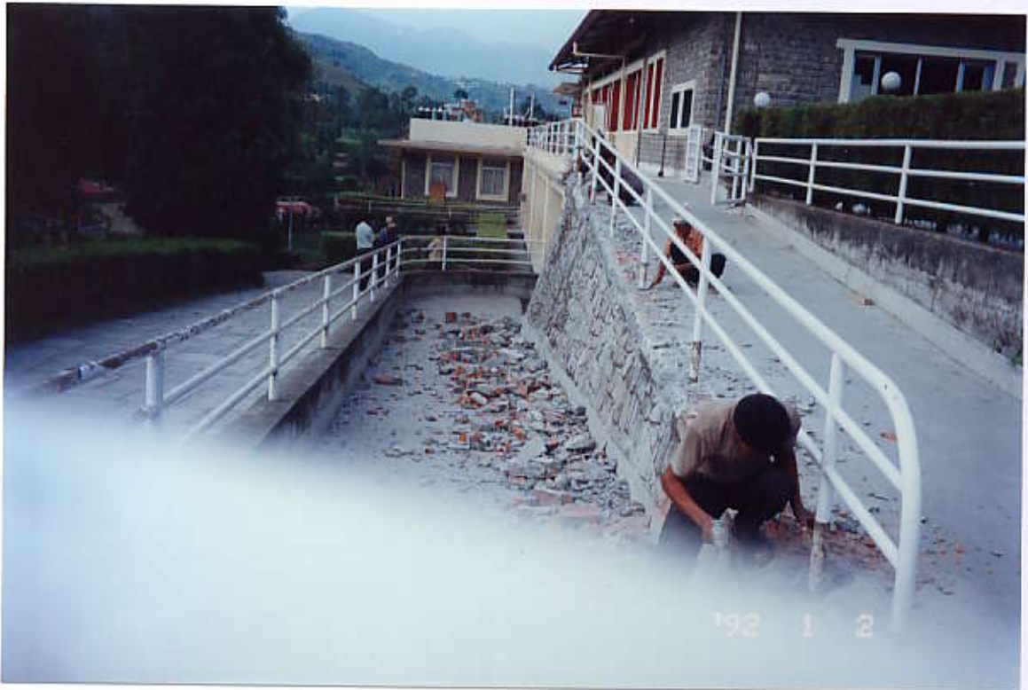
Dismantling of existing side wall of upper Ramp for height extension (View from North Side)
