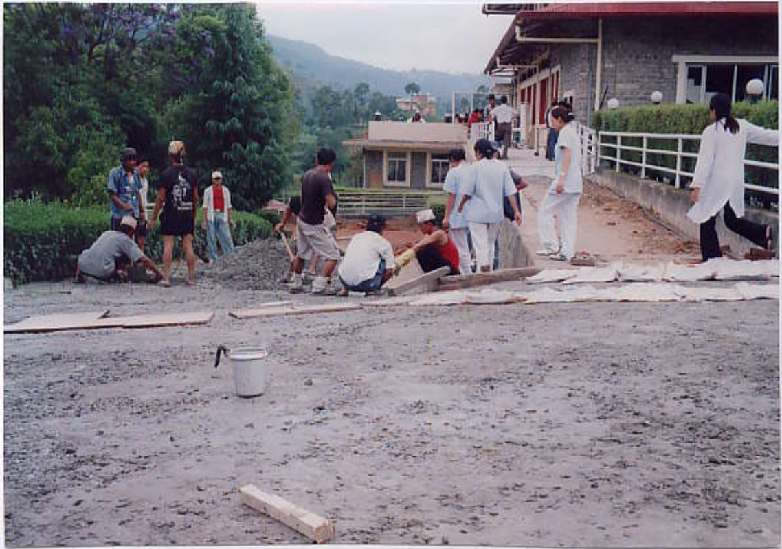
Base concreting for flag stone pavement in progress (View from North Side)
