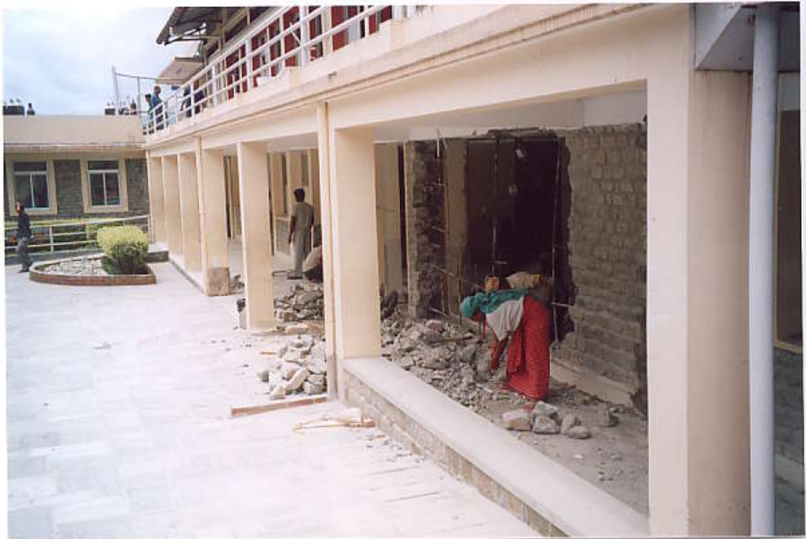
Dismantling some part of existing wall to accommodate new door and large window (up to floor level) in Patients reception and examination rooms (View from North-East side)
