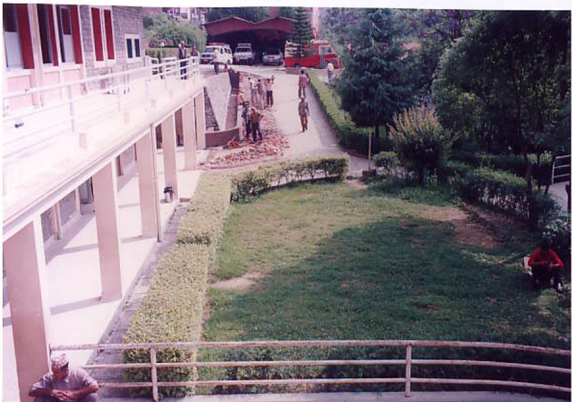
Existing Steel railing at Lower Ramp taken out and back filling on lower Ramp in progress (View from South side)
