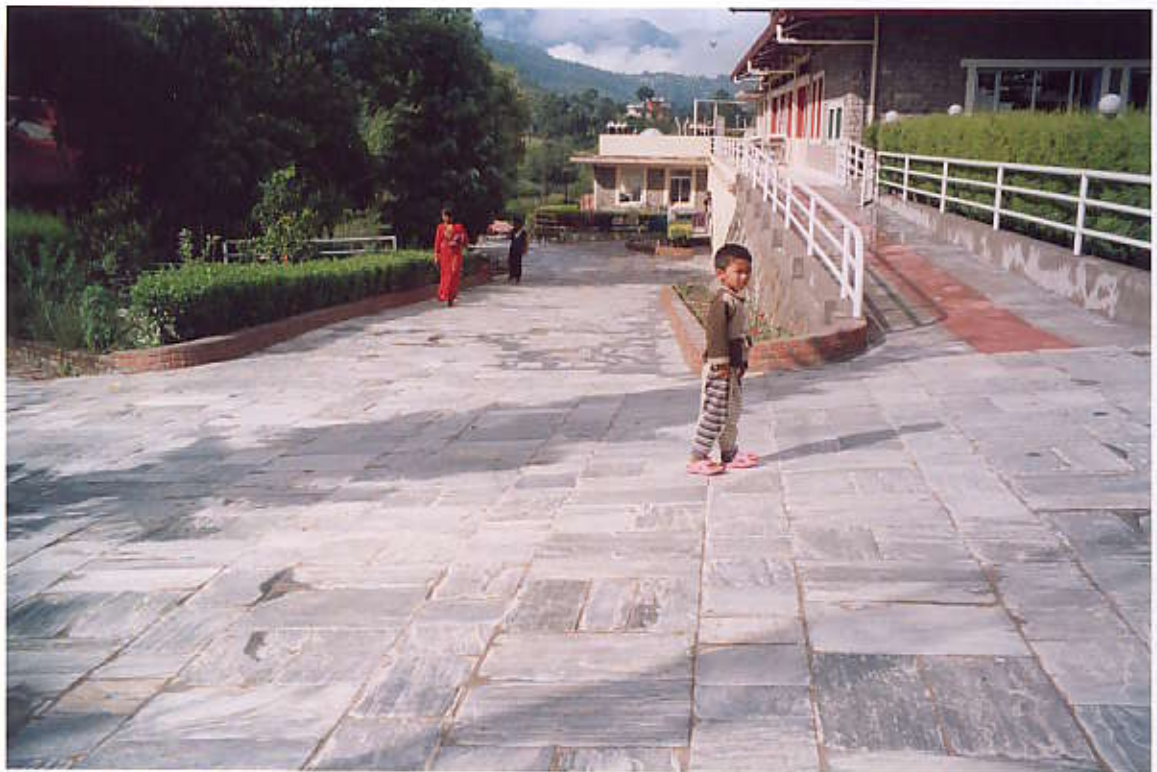
Full view of reconstructed upper Ramp & widened Access Road to Emergency Block (View from North side)
