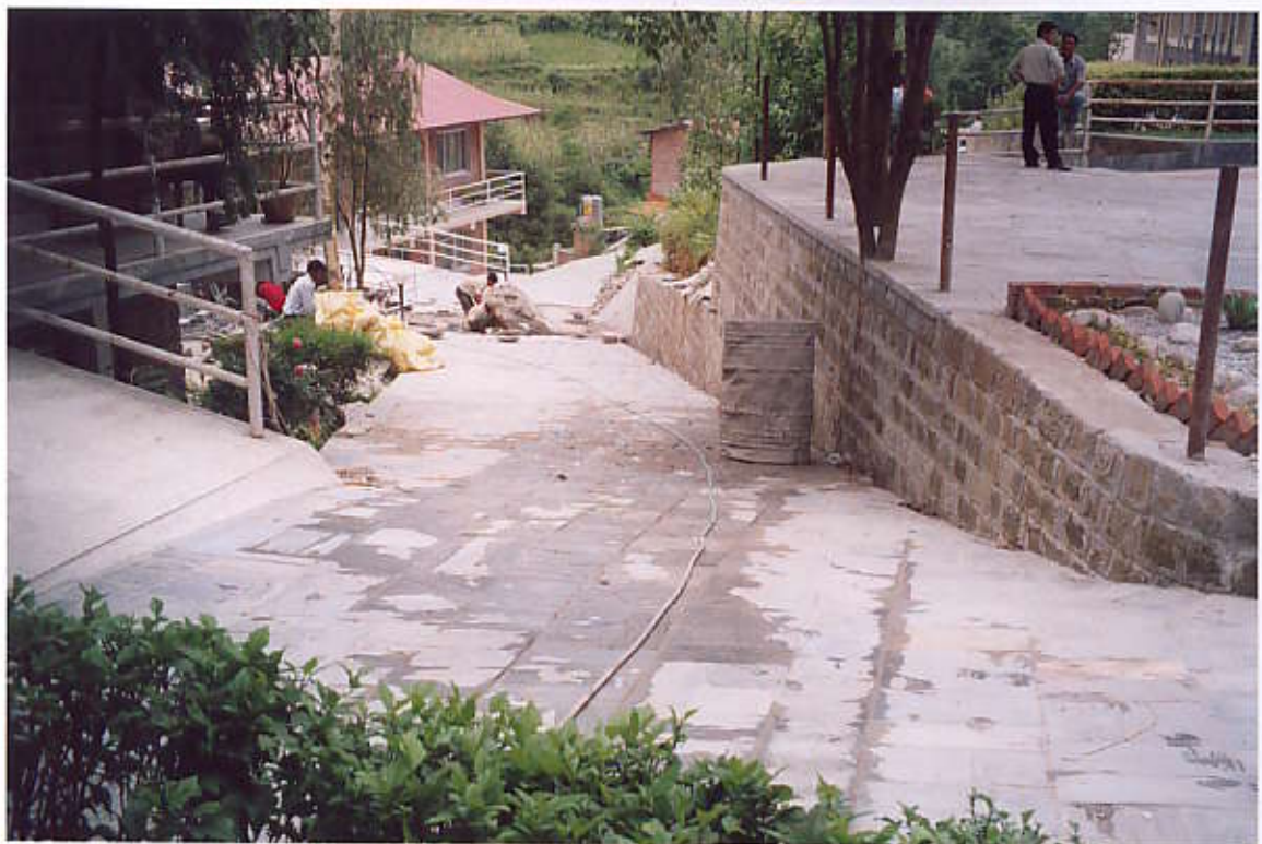
Rehabilitation of existing Access Road to Laboratory Block & Minimally Invasive Diagnostic Department in progress (View from North side)
