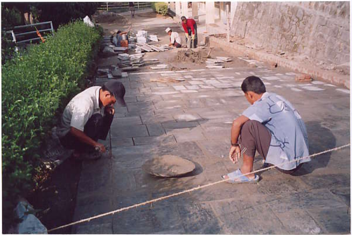
Masons doing cement finishing work on flag stone's joint of widened Access Road (View from North Side)
