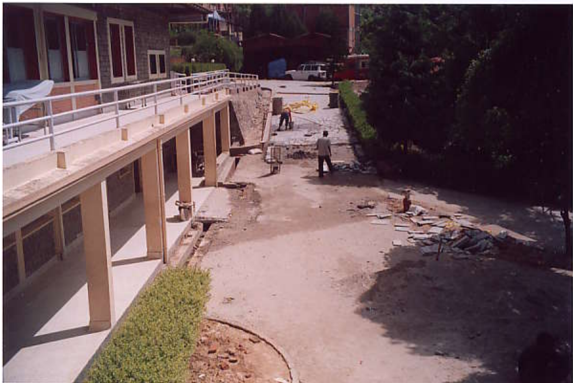
Flag stone pavement on widened Access Road & brick base for Ambulance movement & parking area in progress (View from South side)
