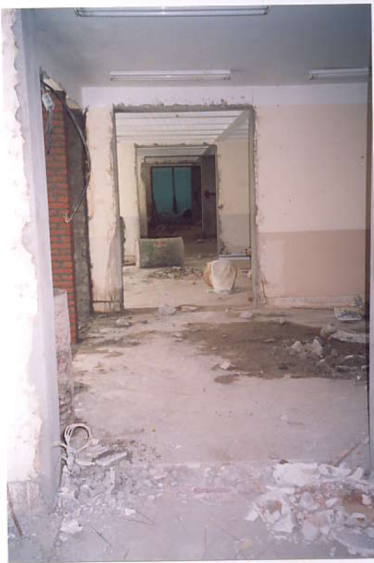
Making of new doors to inter-connect all the rooms of Emergency Block (View from Inside)
