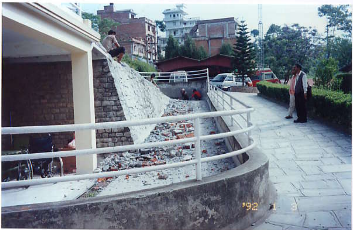
Dismantling of Steel railing of upper Ramp and view of lower Ramp & adjacent Access Road (View from South side)
