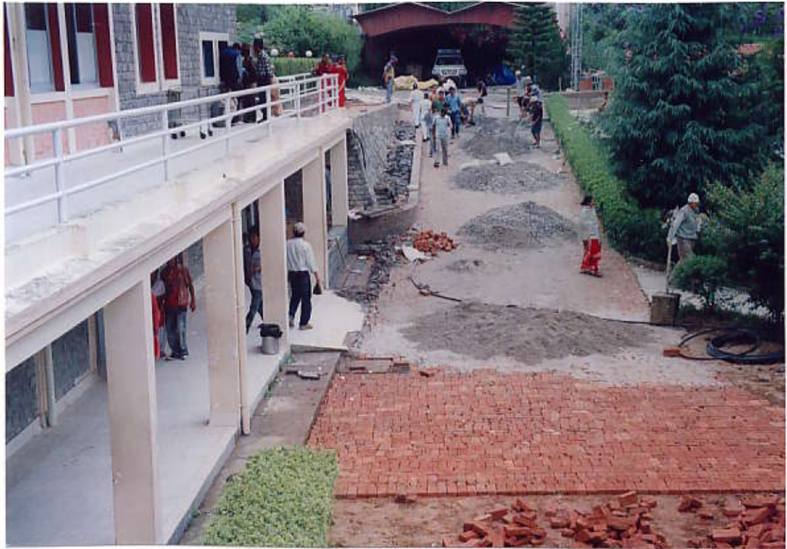
Base concreting on widened Access Road to Emergency Block in progress (View from South Side)
