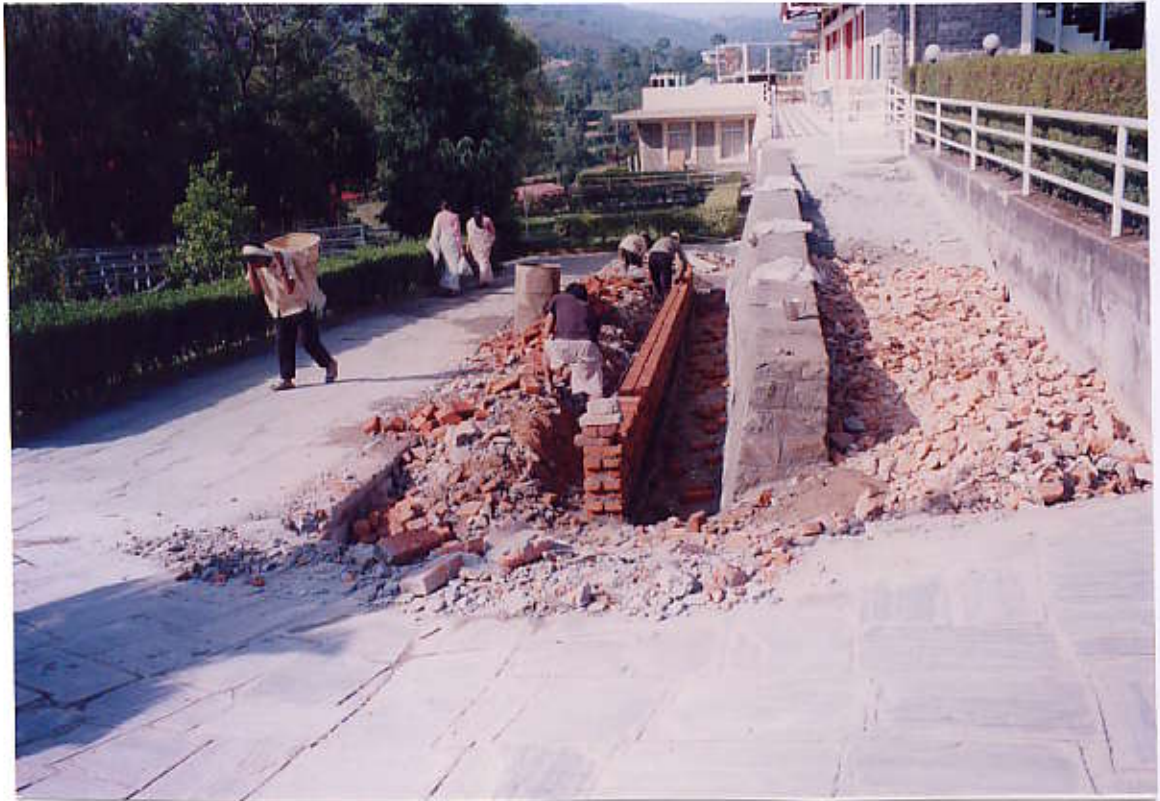
Construction of side wall for flower base and back filling on Ramps in progress (View from North Side)
