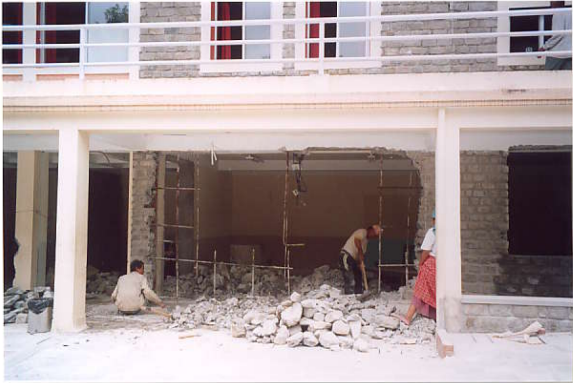
Dismantling of front wall of Patients reception and examination rooms (View from East side)
